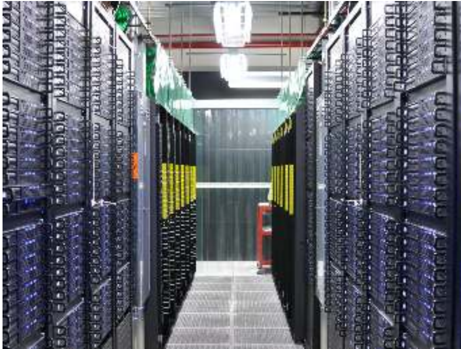
Figure 4. Inside of a data center, showing vertical racks with each rack containing many servers. Source: UL Solutions.
